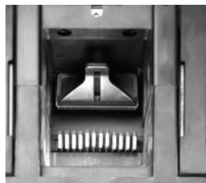
Magnum DS Breaker Contacts (Arc Chutes Removed)
